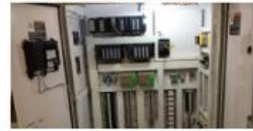
Picture - Panel Internal
